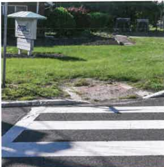
Incomplete pedestrian network at intersection
